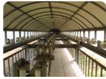
TF, PF, CC & Feeder Jacketing at ASIPP
